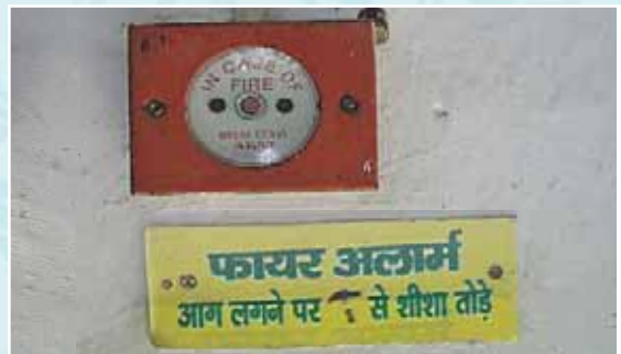
Emergency Fire Alarm Point
